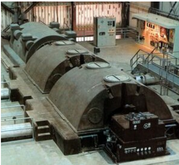
Left: 110MW Geothermal Turbine
